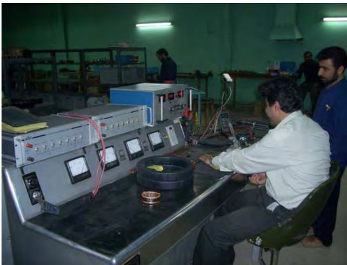
LOW VOLTAGE TEST PANEL
